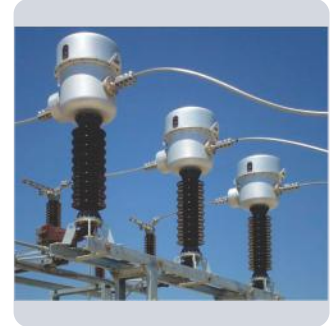
Current and potential transformer
